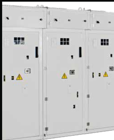
Power Systems and Inverters
